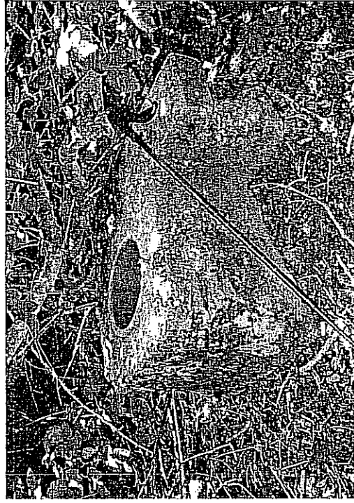
View of the vertical clay pipe and concrete foundation located near the northerly property boundary.
